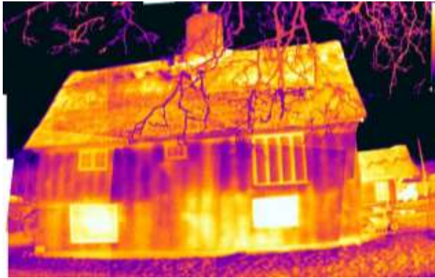
Figure 6. External thermography of east façade. Source: (Author's own, 2017)
