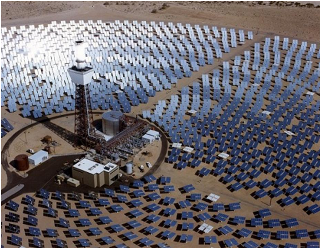
Figure 2.4 Solar power tower surrounded by large number of heliostats, (Sargent & Lundy LL Consulting Group, 2003).
