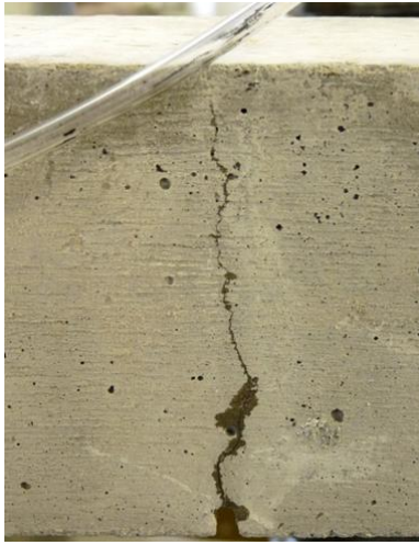
Fig. 5 Twin 1D network showing sodium silicate on crack outer surface.
